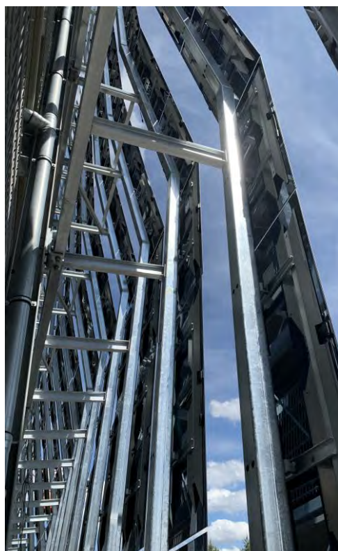
PV-modules on steel substructure
